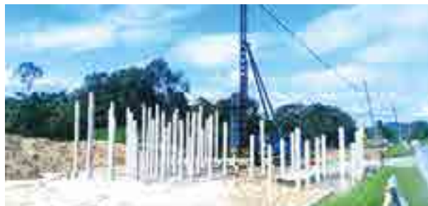
Piling work for Pan Borneo Highway from Sungai Sematan to KSR, Sarawak.
